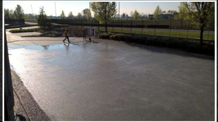
Asphalt clogging with cement mortar
